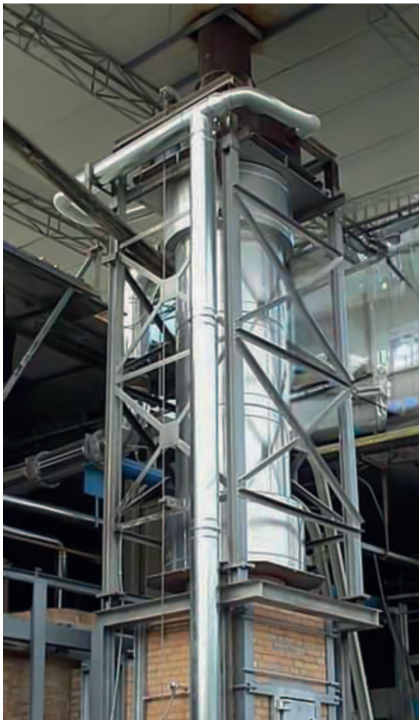
Typical configuration with double stage recuperator
